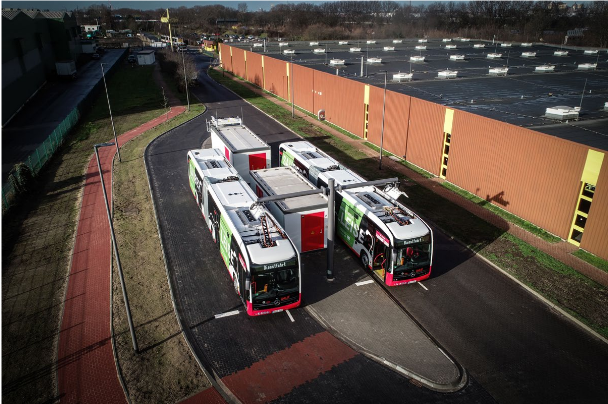
Figure 1: Opportunity charging of two EvoBus eCitaro G at the 450 kW rapid chargers [1] (Image: DVG)
